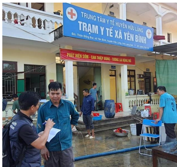
Damaged Yên Bình Commune Health Station, Lạng Sơn Province (Photo: WHO)
