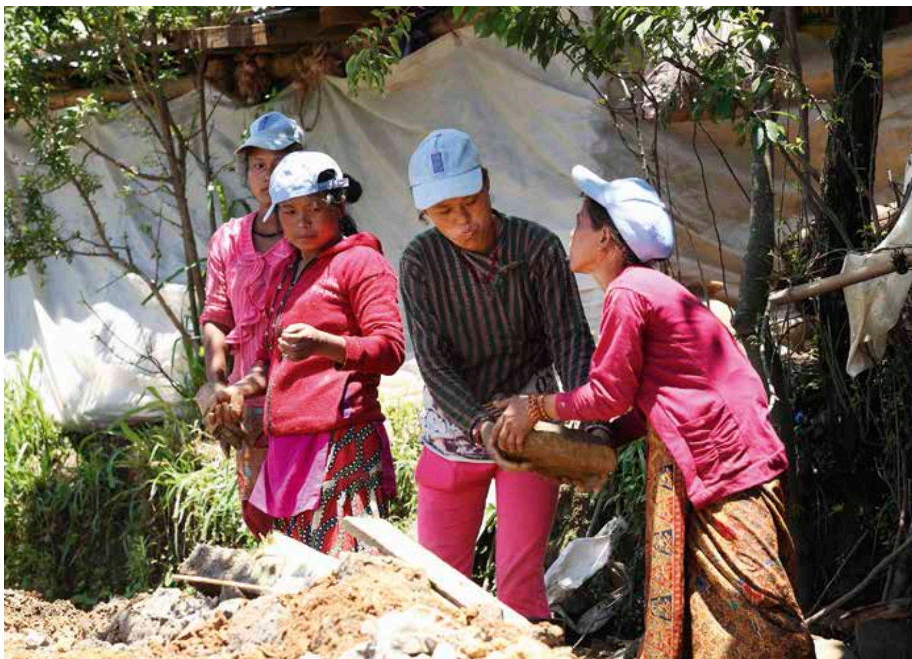
Local volunteers clear debris in the aftermath of the 2015 Nepal earthquake (UNV, 2015).
